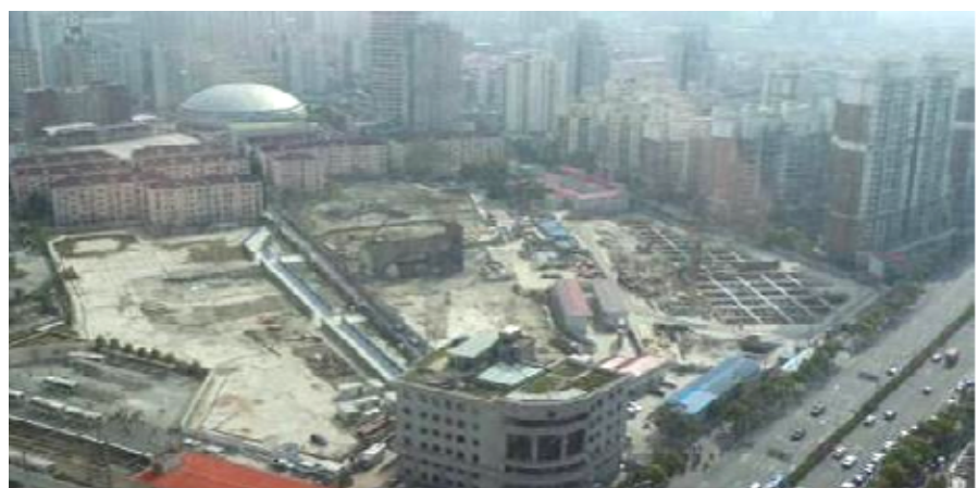
Excavation & shoring system, 14.5% project completion (steel binding and concrete casting) in progress
