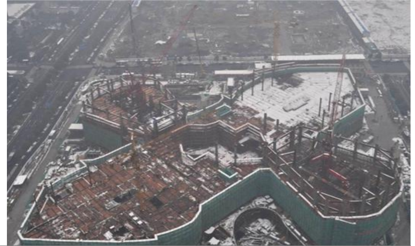
Completion of basement, 20% project completion Reached Level 3 to 4 for both the podium and towers
