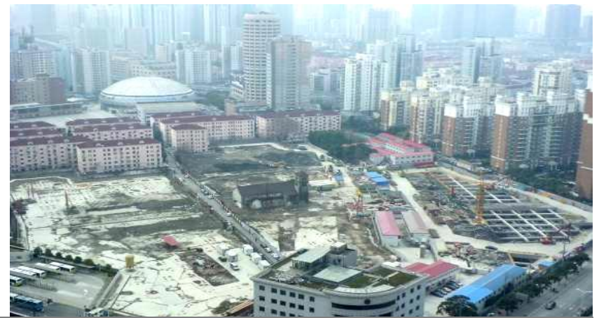
Excavation & shoring system, 12% project completion (steel binding and concrete casting) in progress
